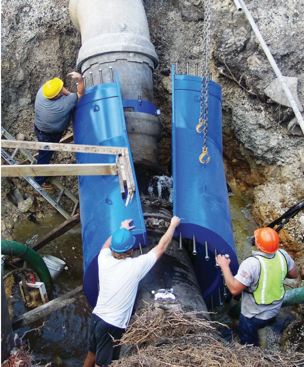
On the left, utility personnel install a Bell-Pack Fitting over failed piping assembly involving multiple existing fittings. This permanent solution was completed in a matter of hours without an interruption to service.
