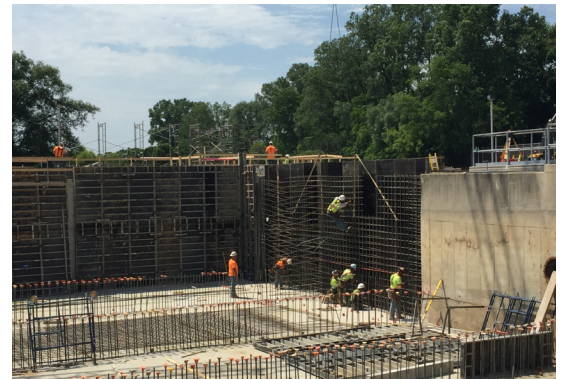
Crews work on construction of a new primary tank during the Zeeland Clean Water Plant expansion in 2016.
