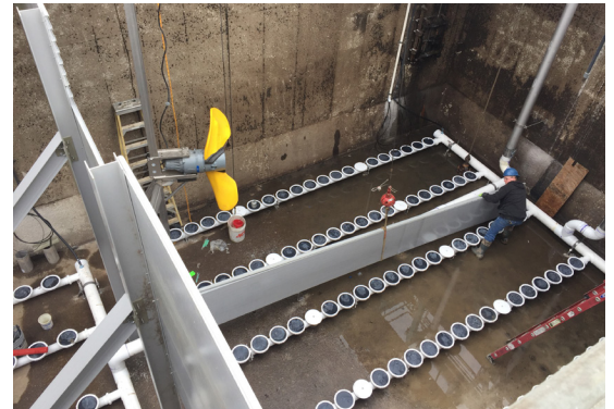
View of a Flygt 4320 mixer inside the tank.
