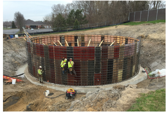
Crews install rebar on a tank during the expansion of the Zeeland Clean Water Plant.
