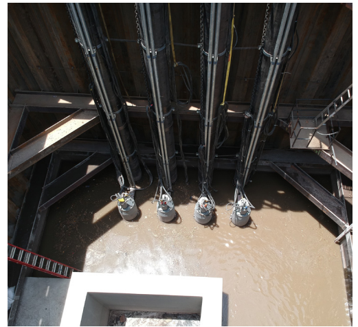
To meet fluctuating flow conditions and address ragging concerns, the Flygt 3531 pumps were mounted on a slide rail system.
