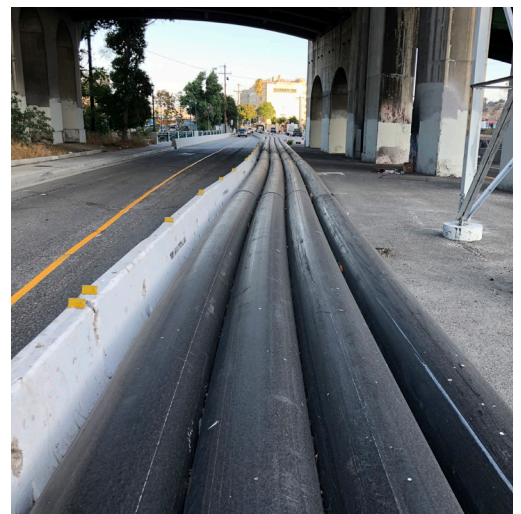
Four 2,500-foot lines of 24-inch HDPE pipe run from each pump to an alternate line located 24 feet away discharging into the Northeast Interceptor Sewer.
