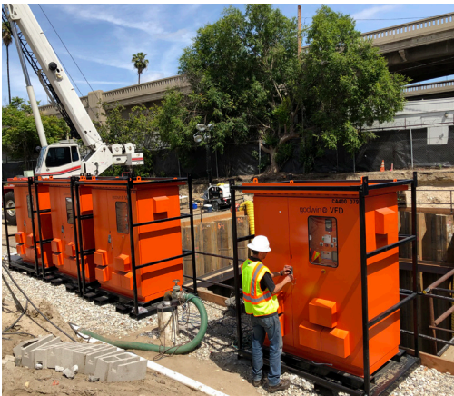
Godwin variable frequency drives (VFDs) optimize energy consumption and allow the pumps to automatically start and stop to maintain a consistent sewer level.
