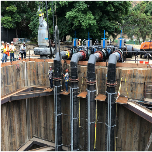
A 35-foot suction pit was excavated to stage Flygt 3531, 335HP, 24-inch electric submersible sewage pumps.
