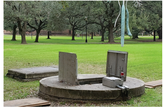
Baker Institute lift station.
