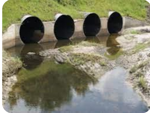
No Storm Water drain data
