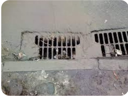
Poor Storm Water Drains
