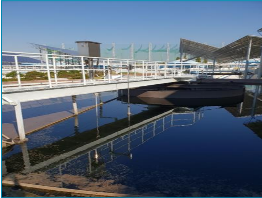
South Korea Suwon WWTP
