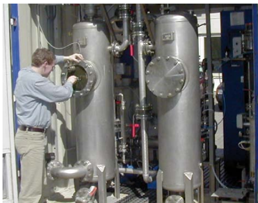
Fig. 6: Ozone pilot plant
