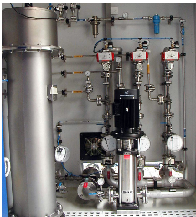
Turnkey containerized WEDECO ozone system incl. triple injection system.
