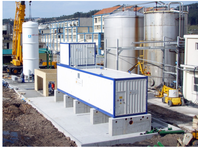
Build-up phase of the containerized WEDECO ozone systems incl. liquid oxygen storage
