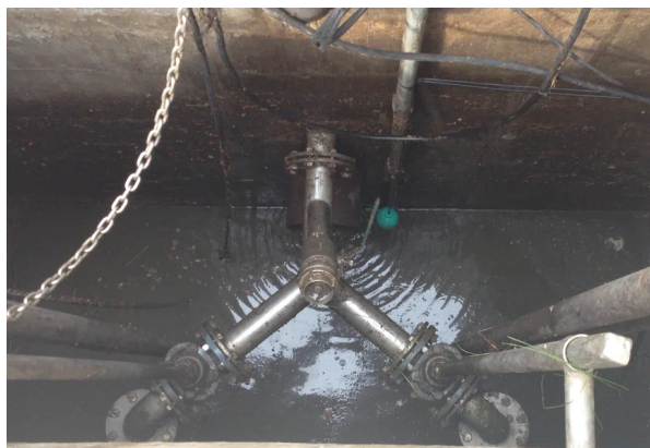
A view of Flygt's clean pump sump after installation at the pumping station
