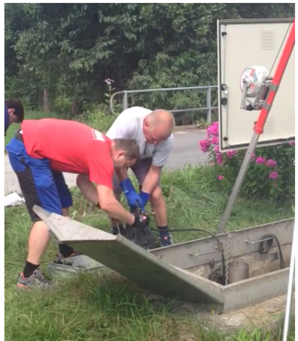
Xylem's Flygt Concertor is installed at RHV Mühlthal, Austria
