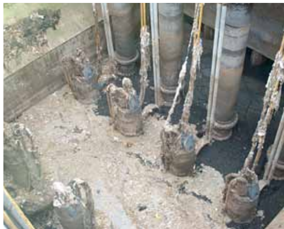
Pump station with accumulation of floating debris.
