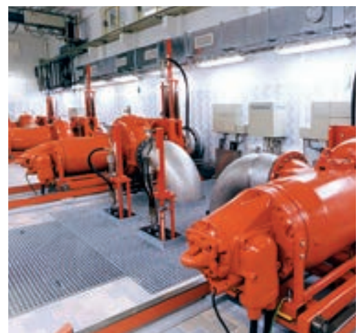
It isn't every day Flygt pumps get painted red. That's what the architect stipulated when the Karl XII pumping station in Stockholm was built.
