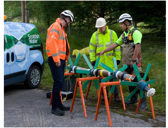
Preparing the PipeDiver platform to inspect the Newmore Raw Water Transmission Main
