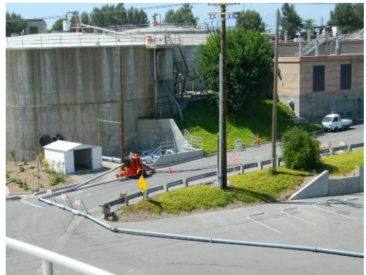
Digester being dewatered to waste backwash lagoon.
