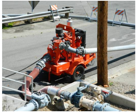
NC150 Dri-Prime pump takes suction from pipeline that connects to bottom of digester.
