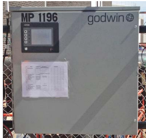
The Godwin 450 HP variable frequency drives also installed on site are connected with the plant's own SCADA system, custom-developed by Xylem.
