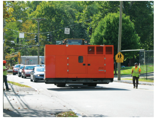
Although the project was located on a heavily traveled road near a major interstate and local businesses, setup of the system went smoothly.
