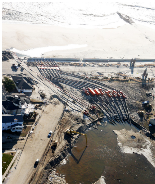
The outfall structure of Lake Como in New Jersey was compromised by Hurricane Sandy. Eight Godwin Dri-Prime CD400M pumps and two CD225M pumps were installed to route water to the ocean during future rainwater storm events. Photo courtesy of Star News Group.
