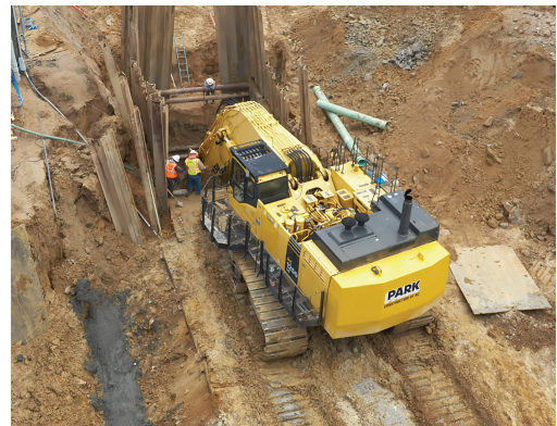
The temporary sanitary sewer bypass system in Raleigh, North Carolina, allowed the city to replace a major outfall line feeding the city's wastewater treatment plant.
