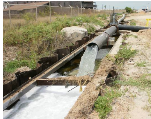
Tee to divert silt-free water back to bay or water containing silt to the retention pond.
