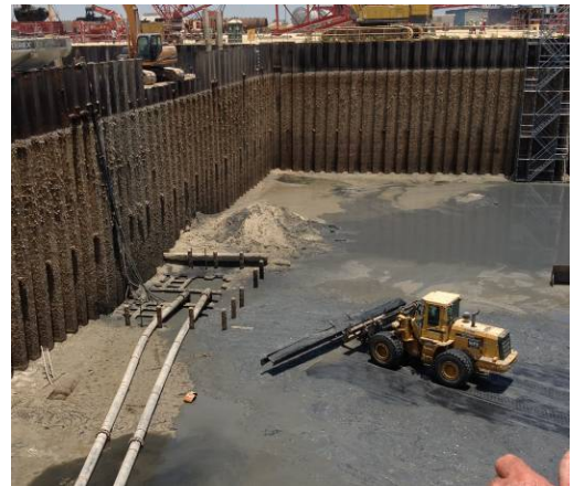
Customer is pushing silt from bottom of the structure to the sump area. Pumps will remove excess water and silt to retention pond for disposal.
