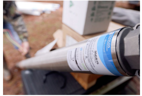
Crews installed a Goulds Water Technology 35 GPM, 7.5 HP submersible pump and motor in the new 720-foot well.
