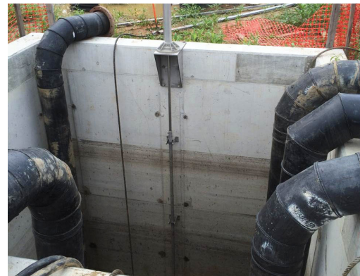
High-density polyethylene pipe exiting the wet well.
