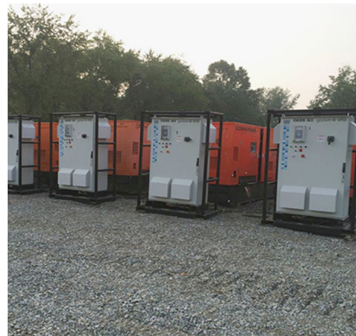
As part of the rental solution, Godwin VFDs and Generators - one set for each of the five Flygt pumps - were integral to the bypass operation.
