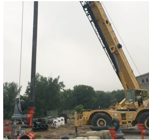
Once the piping was affixed to the Flygt pump, it was lowered into the wet well.
