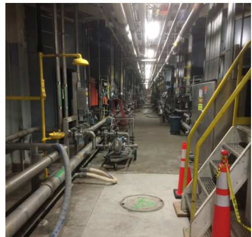
Inside the facility, the tight spaces were a challenge for running hose and for suction-point access.
