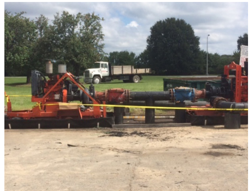
Two Godwin diesel-driven CD225M stainless steel pumps in place for the external, sewer line bypass.
