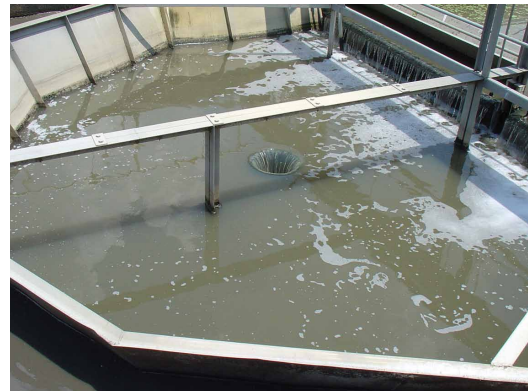
Before: The plant's five floating mixers/aerators could not deliver enough oxygen or mixing.
