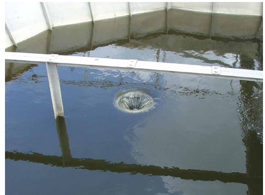
After: Since completion of the retrofit, the plant operates with just two new mixers and has visibly better results.
