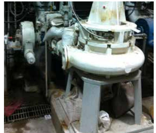
BEFORE: Sand bags were placed on the pumps to decrease vibration
