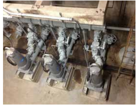
Closed loop cooling of the motors eliminated seal water piping, seal pots and the compressor
