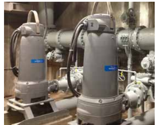
AFTER: Standard air cushioned check valves and Pumpsmart VFD's allowed for the elimination of the old style hydraulic oil operated valves decreasing complexity of the system
