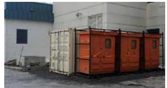
VFD Panels outside of RSPS
