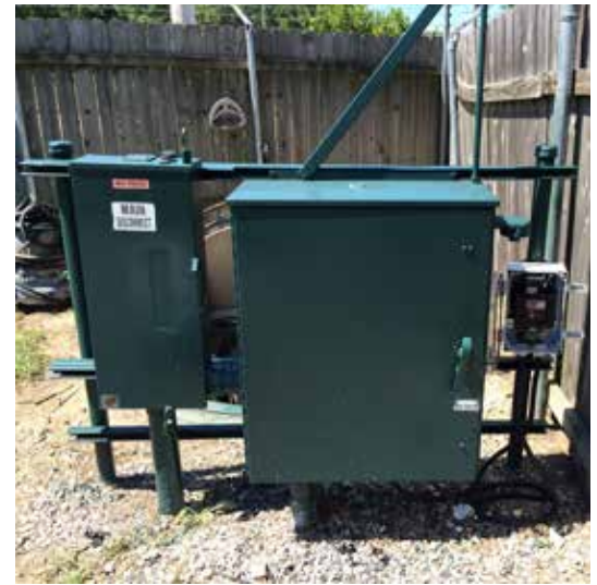
Existing control panel next to Concertor control
