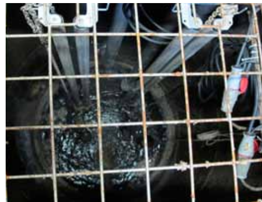
A cleaner pump, sump and pipe means less odor, reduced labor and maintenance costs.
