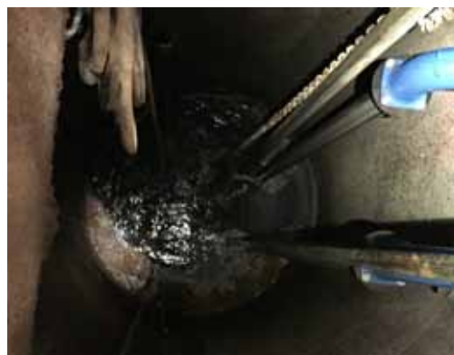
New pump in the wet well
