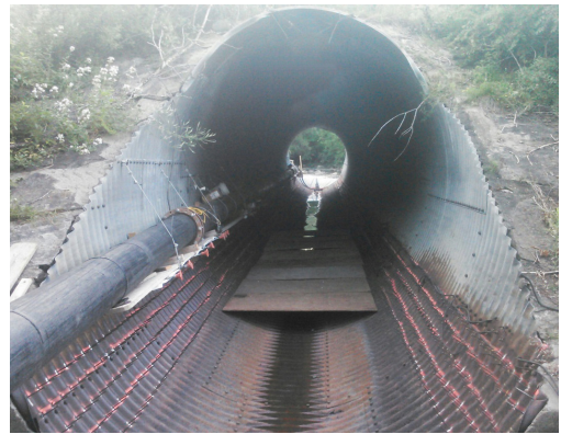
The DH Smith solution required a complete temporary bypass, with the piping passing through the culvert and rigging to hang the pipe off the side of the culvert.
