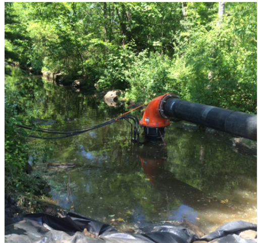
The Godwin Heidra 600AX Axial Flow dewatering pump provided enough flow capabilities to move the Mayfield Creek water from one end of the culvert to the other.
