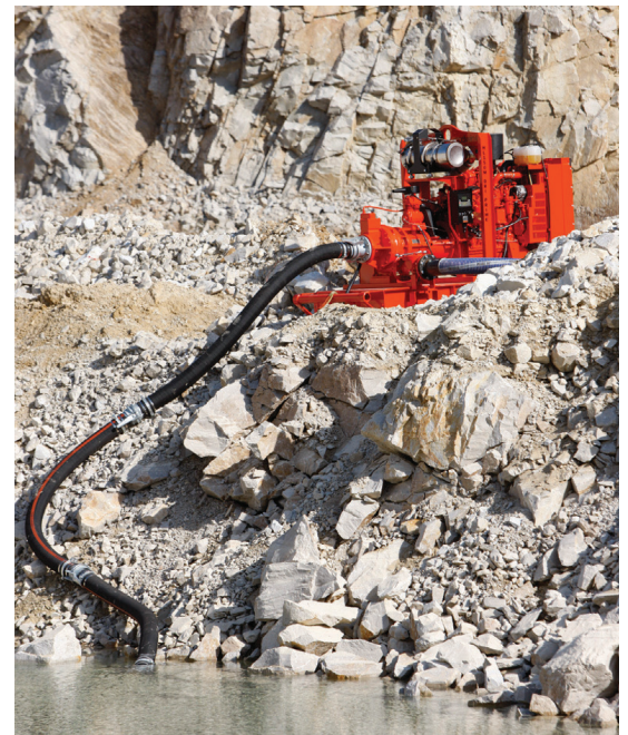
A remote monitoring system that includes Godwin Dri-Prime pumps helps this operation in Perú drain water from an open-pit copper mine.
