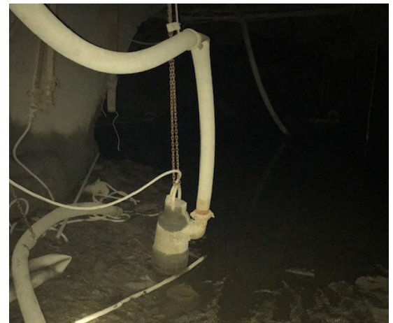
Mine slimes had built up in the sump before Flygt mixers and pump were installed.
