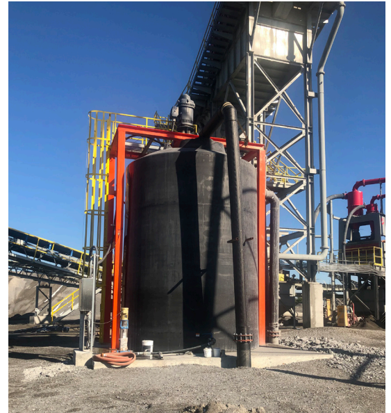
A Goulds Water Technology e-SV 5 stage stainless steel multistage pump provides water to the 200 trees planted by the customer to create a sustainable barrier between the road and plant, complementing the local environment.
