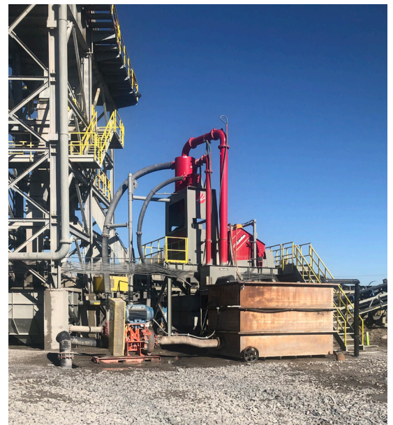
As part of our turnkey solution, a slurry pump was installed to pump 3000GPM of water and fine material through 1600 feet of 12 inch SDR11 HDPE. This pump is robust and reliable, capable of pumping this harsh material with minimum maintenance required.
