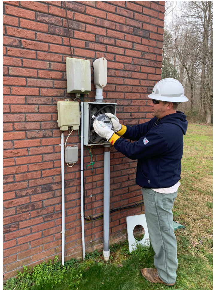
EnergyUnited AMI Technician Terry Lippard installs a new Sensus Stratus meter as part of the co-op's modernization efforts to enhance member service.
