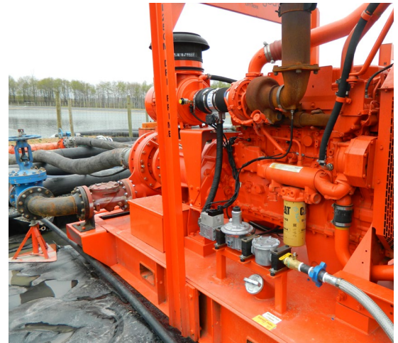
Godwin HL250M dual fuel pump engine integrated with Xylem Advanced Remote Monitoring (ARM) technology significantly enhanced the sustainability and efficiency of the project's water transfer operations, saving approximately $25,000 per month in labor costs as well as revealing the benefits of switching to a dual fuel pump engine.
