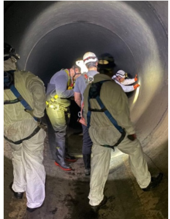
The Xylem team is pictured performing a visual and sounding inspection of the pipelines. This provides an additional data set to compare with information collected during an electromagnetic examination, and increases confidence in the location and presence of wire breaks and significant pipe wall deterioration.
