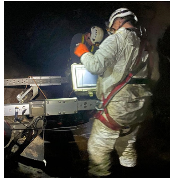
The Xylem team is seen here performing a manned PipeWalker electromagnetic inspection of the pipelines. This provides high resolution condition data about the pipe wall and prestressing wires.
