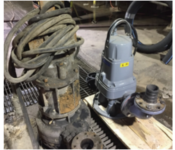
The original 7.5 HP submersible pumps (left) were replaced with the smaller yet more powerful 10 HP Flygt Concertor.
