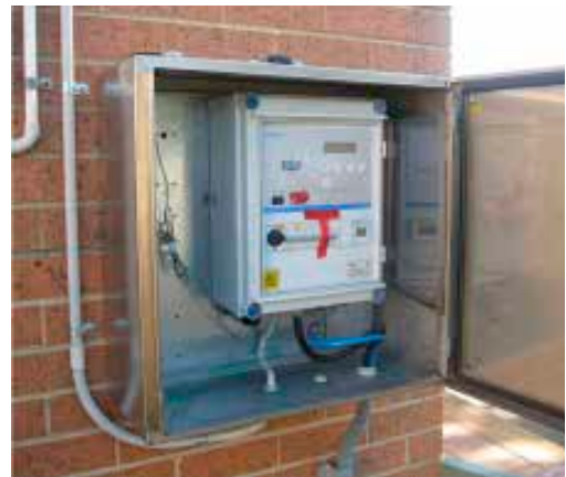
Controller at Tooradin Comfort Station.
