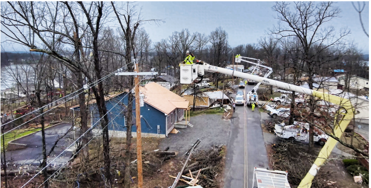
The resilient infrastructure allowed West Kentucky Rural Electric Cooperative and mutual aid crews from neighboring states to kick off a targeted restoration effort following the weather emergency.
