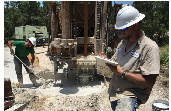
The team from H.M. Schwoppe & Sons works on completing the installation of the new well.
