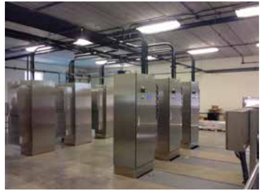
State-of-the-art stainless steel and air-conditioned ballast cabinets providing the power to the UV disinfection system
