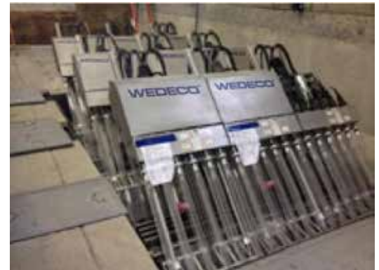
Wedeco Duron UV disinfection system installed in the Rensselaer County Sewer District water treatment facility
