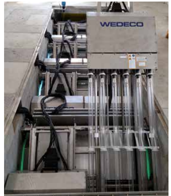
A 12-lamp module of the Wedeco Duron UV system that has been raised by the automatic lifting system and is ready for maintenance.
