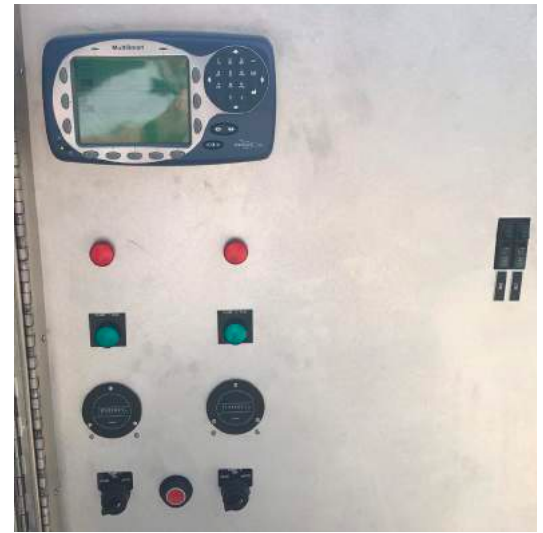
The MultiSmart IPSM with touch screen collects more than 400 sophisticated data points at each site for Lowndes County.
