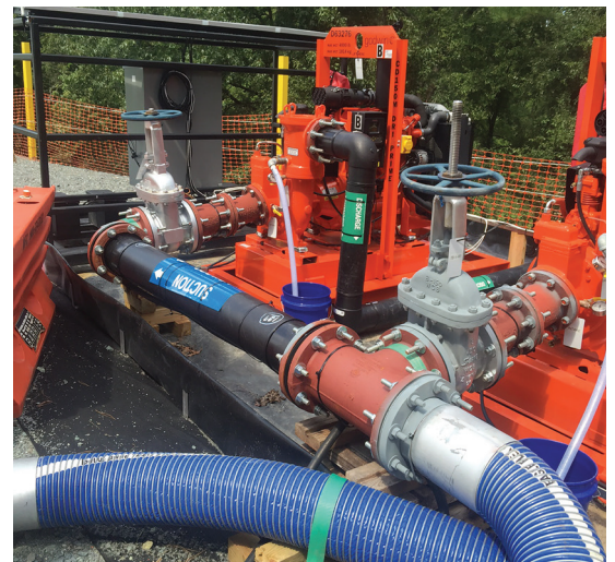
Due to space limitations, Xylem engineers designed a pad layout incorporating a common suction line for this particular site application.
