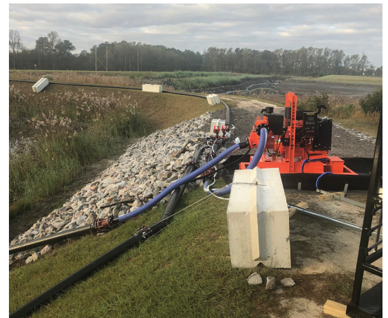
Godwin diesel powered pump used to remove ash pond water from clear pond and pump to outfall with Xylem pre-treatment control system ensuring water being discharged meets site permit limits.
