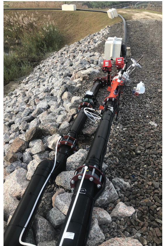
Chemical injection points, flowmeters and automated valves along the Xylem pre-treatment system to operate without the need for an operator.
