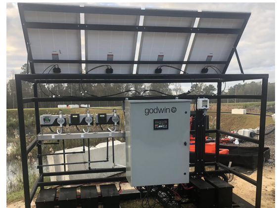
Xylem custom control panel with solar array and chemical injection pumps at remote ash pond site.
