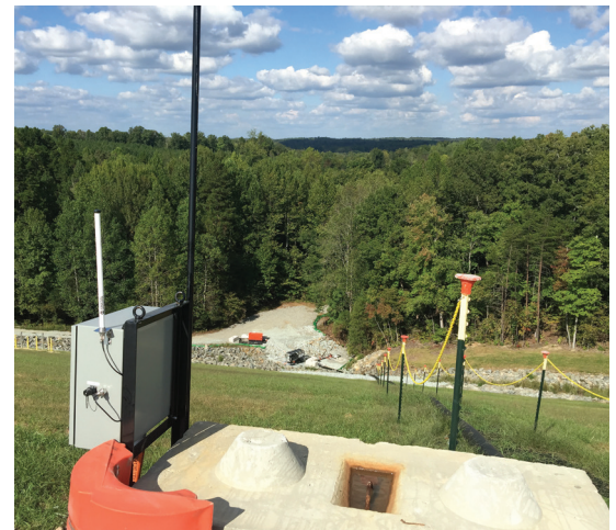
View from top of ash pond dam at discharge point looking down at seep collection site as base.
