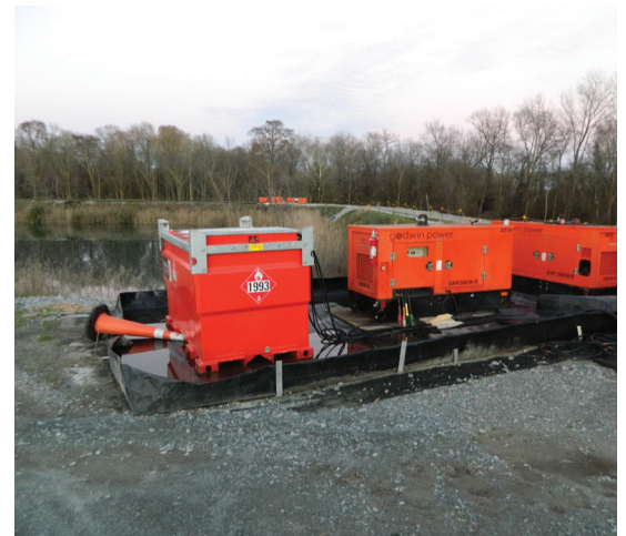
Rental external fuel cell along with two generators provided extended run times between refuel and allowed for service of equipment without system being offline.
