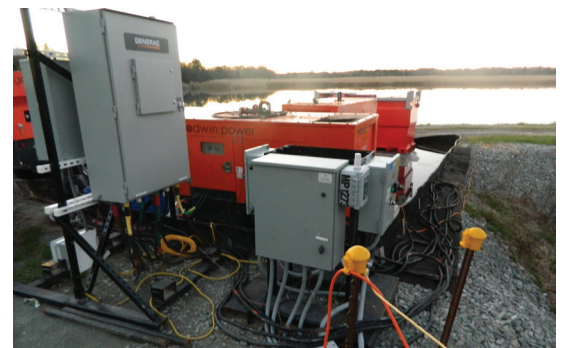
Rental transfer switch and PLC controller allowed for 24/7 operation of this system and provided back-up in the event equipment needed to be repaired or serviced.
