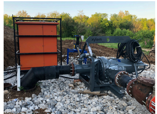
The Xylem team used a horizontal, dry pump installation for the Flygt N 3312 pump.
