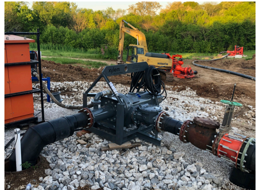
The custom-engineered pump and priming system operated at the temporary bypass site for eight months.
