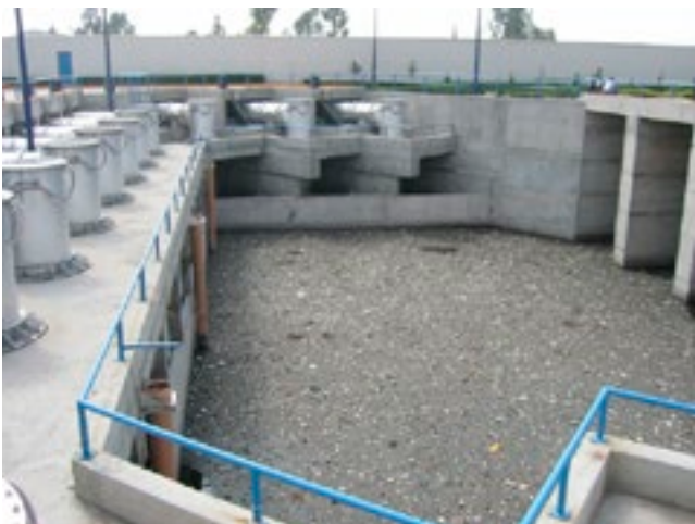
Example of a typical wastewater station with propeller pumps.
